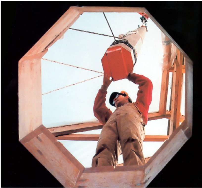
Figure 26 - The framed, octagonal opening through the quarterdeck waits to receive the mizzen mast. The mizzen was the first of the Kalmar Nyckel's three masts to be stepped in the day-long process which moved from aft to fore. Photographer – Chris Queeney.
